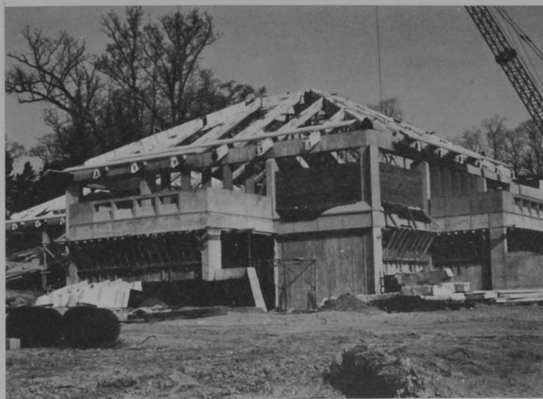
KENYON'S NEW women's commons finally begins to take shape as work continues on schedule.
