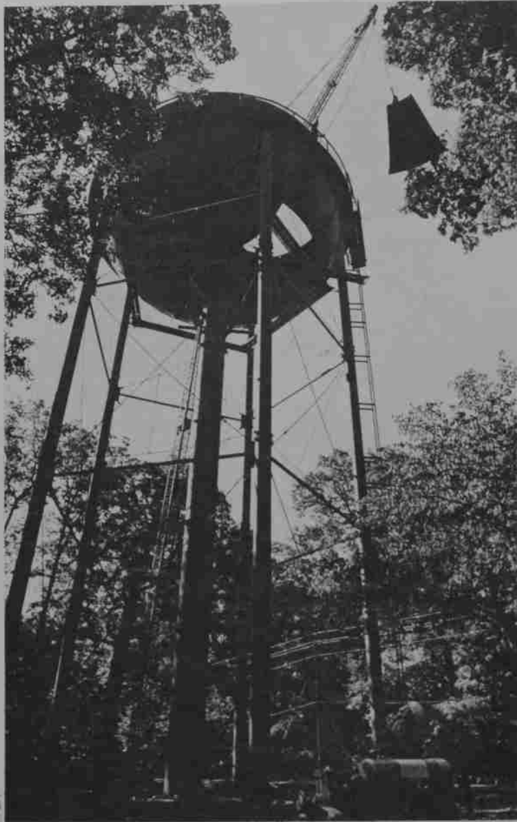
Progress on Gambier's new water tower indicates that the forecast is "all systems go" as winter rapidly approaches.
